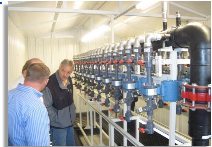
Interior of Ur-Energy's prototype Header House
