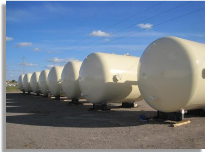
Ur-Energy's Ion Exchange Columns
